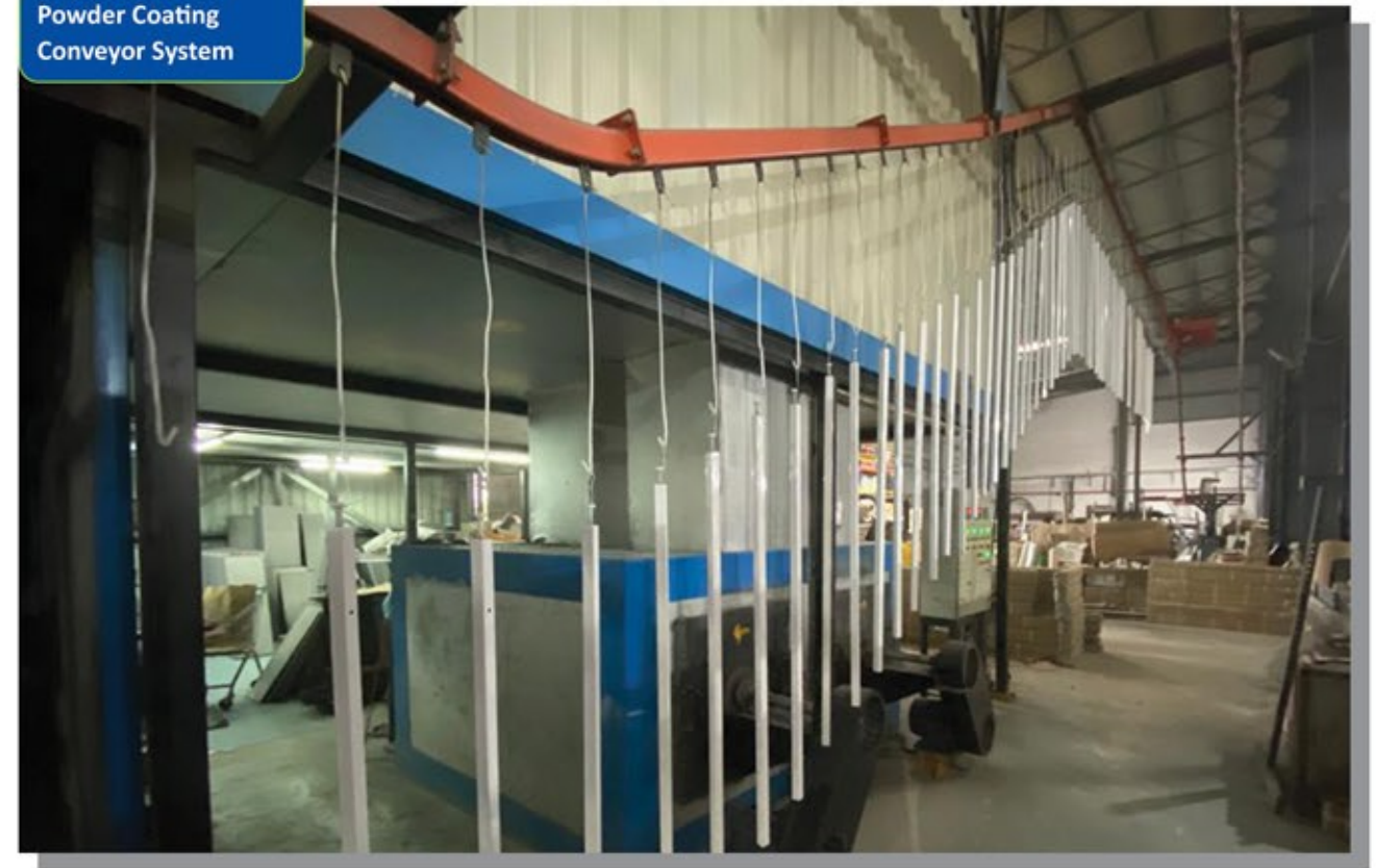
Powder Coat Spray Booths With Conveyor System
